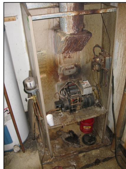
Figure III-12. Fuel Oil Forced Air Furnace in Wainwright (approximately 30 years old)
