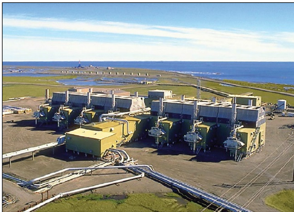
Figure III-5. BP Central Compression Plant
