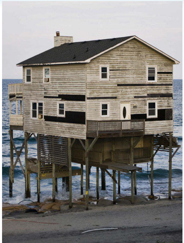
This house in North Carolina was condemned due to beach erosion along the Outer Banks (Nag's Head). Photo by Artcphotos/Shutterstock.com.
