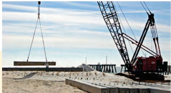
Constructing the new Gulf State Park Pier, Gulf Shores, Alabama. Photo courtesy of Alabama State Parks.
