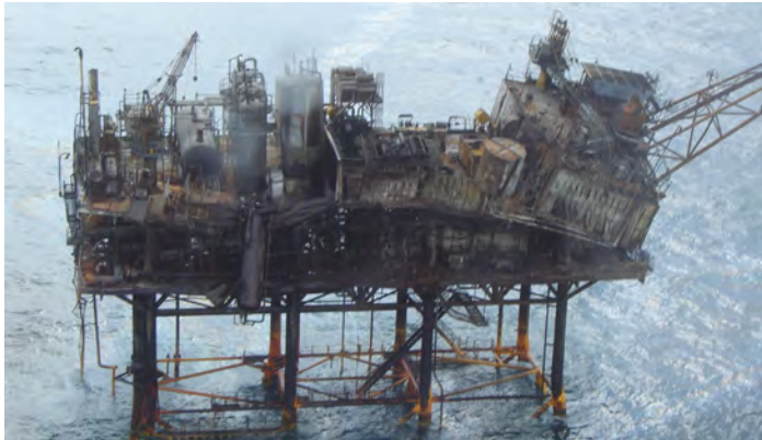
Eugene Island 296 E platform, in the Gulf of Mexico, which burned due to damage from Hurricane Ike in September 2008.
