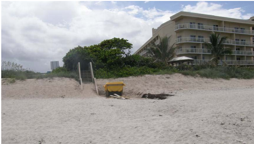
Figure 2-18. Existing storm water outfall drain near Howard Futch Park, south of Crowne Plaza hotel (monument R-109.2)
